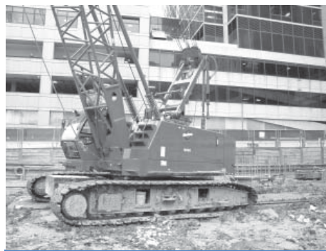
Manitowoc Crane fitted with DOC at Yawkey Center for Cancer Care Site
